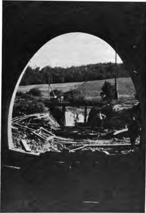
PLATE 64.—View of South Portal of Peak Tunnel, Looking from Interior of Completed Cut-and-cover Aqueduct.
